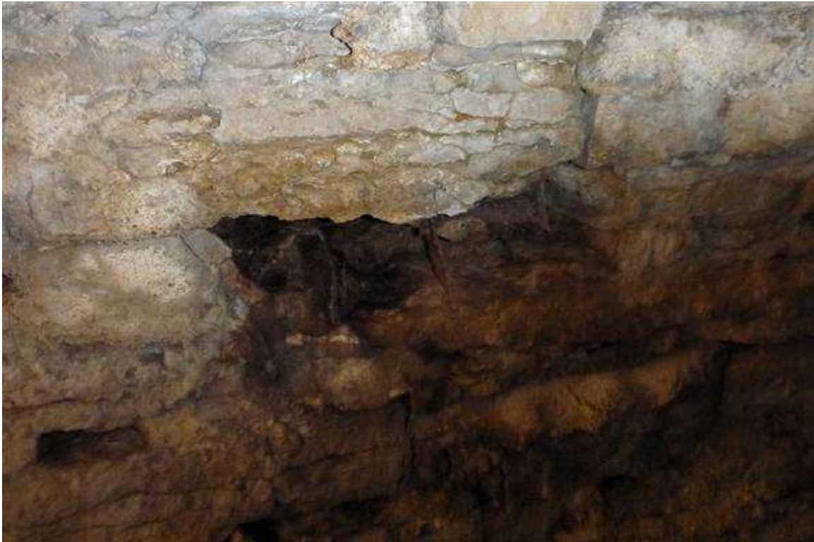
Photo 2 - missing stones near West Headwall
