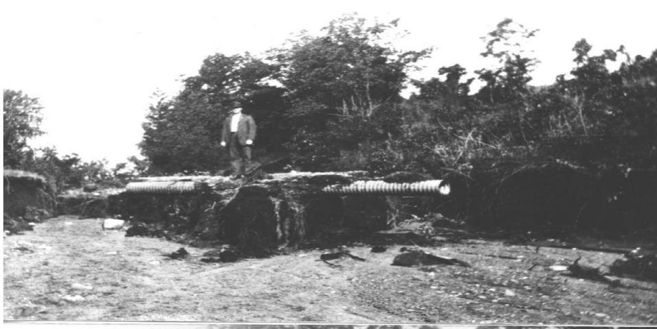
Erosion of roads after storm event exposes drainage pipe. Image source: Afton Historical Museum. (Add image ID #)
